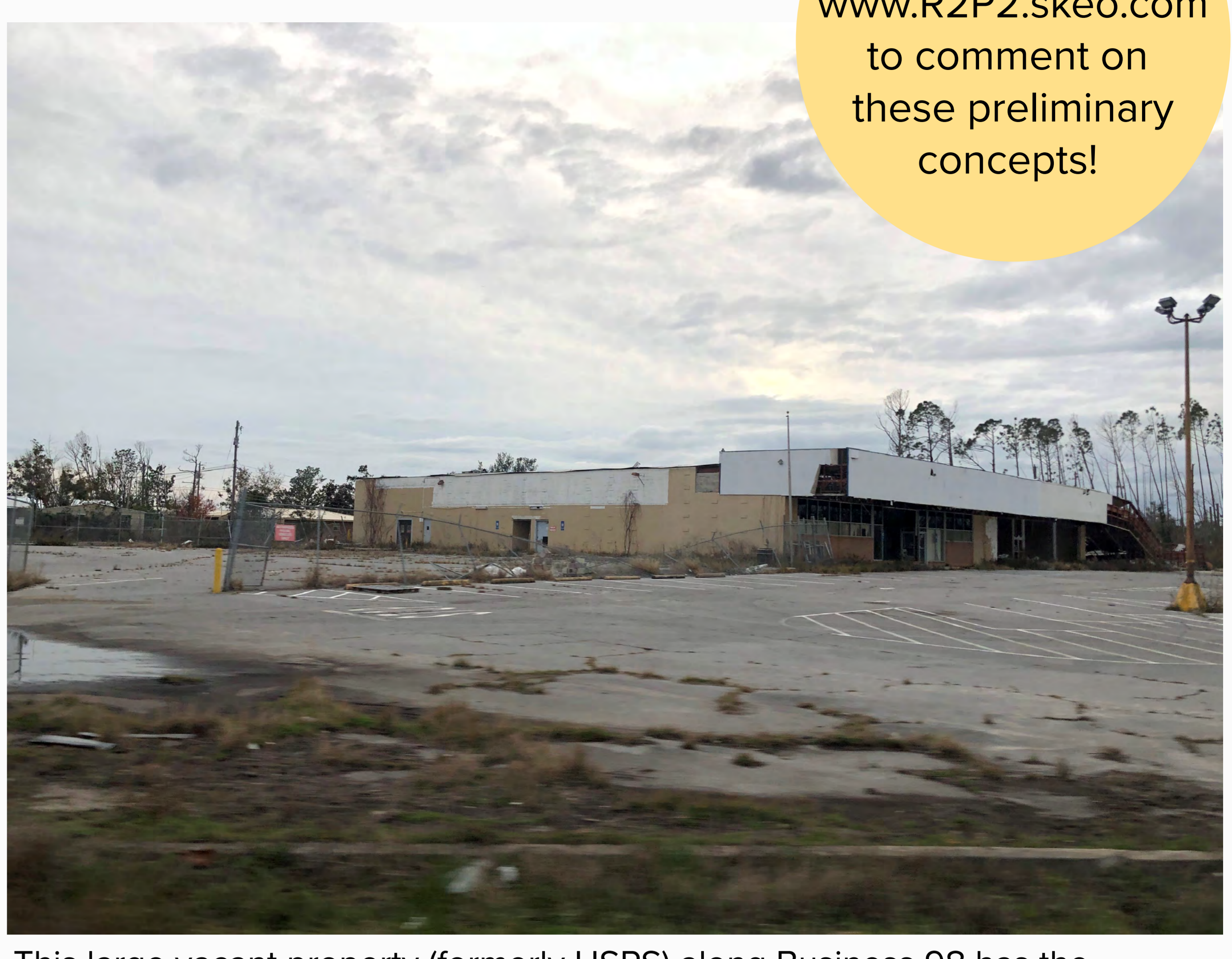
This large vacant property (formerly USPS) along Business 98 has the potential to become a catalyst for mixed use development along the east end of Parker.
